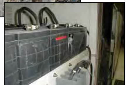
Thermal runaway incident
