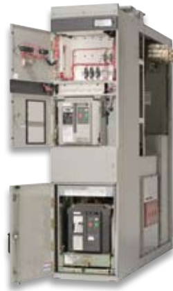
Integrated Unit Substation
